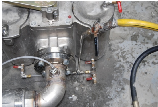
Figure 7 - Fresh Water Fill Line to Suction Strainer
