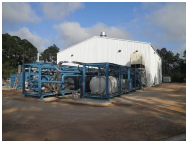
Figure 5 Installation pictures of the 10.5 TPD PRR system
