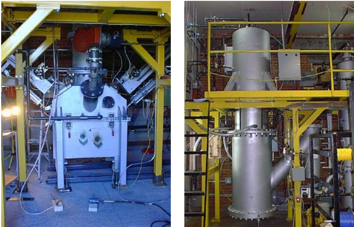
Fig. 2. View of the pilot plant: PAGV furnace (left) and off-gas treatment equipment (right).
