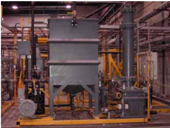
Figure 6 Pilot PRR System Syngas Cleaning Skid
